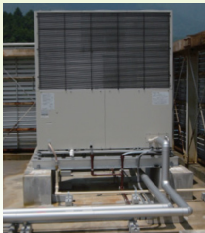
Installed Gas Heat Pump on the No.3 Building rooftop
