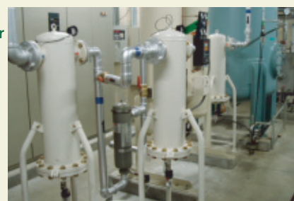
Pre-filter and after-filter
